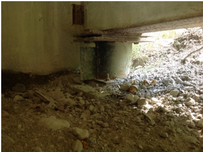
left bank pipe risers - typical
